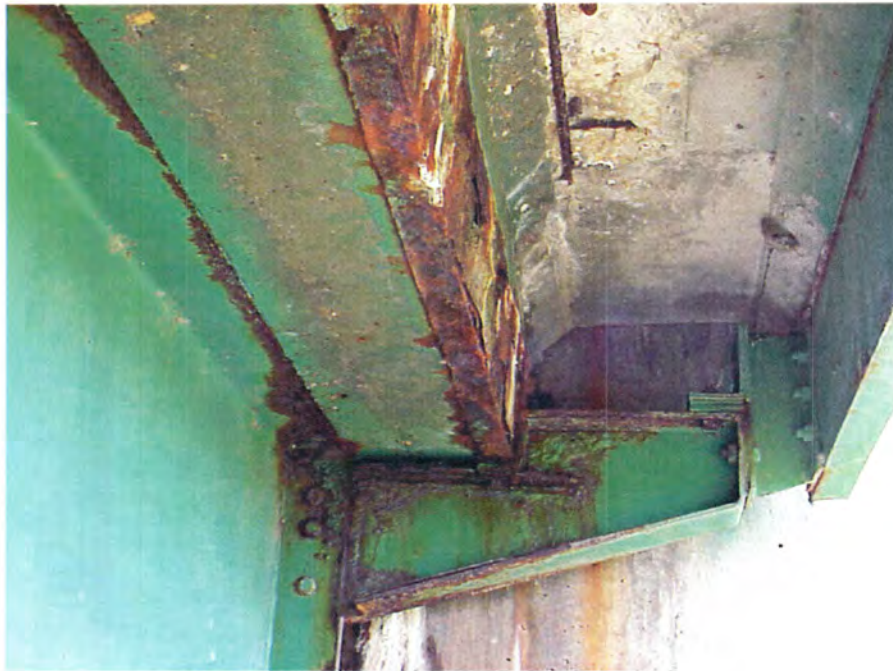
(e) Typical condition of deck soffit and deck channel Figure I-1. Overall bridge photographs - continued.
