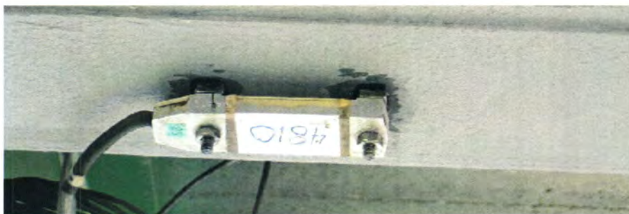
(b) Photograph of typical strain gage installation on CFRP plate Figure II-25. Strain gage location for "Shortly after installation" test.
